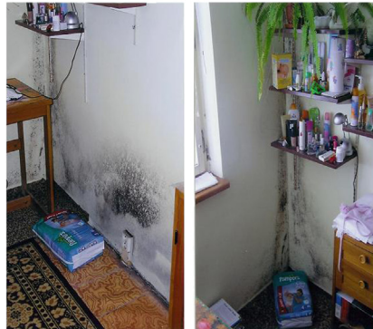
FIGURE 10 Severe mold growth on walls as a consequence of thermal bridges with the critical surface temperature < 12.6\text{ }^{\circ}\text{C} at RH > 50\% . Statistical probability of undesired fungal colonization at p < 0.001 .
