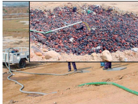
Photo 2-8 Leachate recirculation treatment system at a landfill in Mexico City
