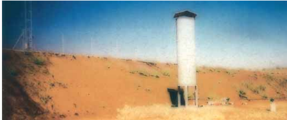
Fig. 3.11d Connections for biogas and flare stacks.
