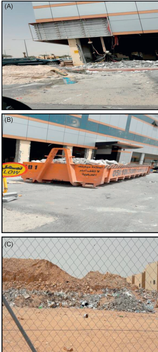
Figure 2.22 (A) Construction/demolition sites maintained neatly; (B) carrying demolition/construction material; (C) dumping yard far from city.
