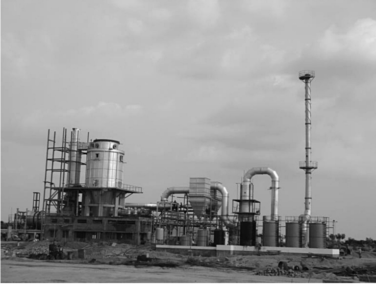
Figure 5.19 A large capacity hazardous waste incinerator.
