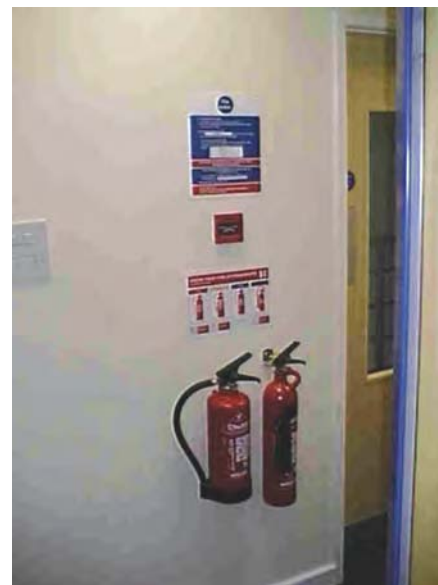
Figure 11.9 Typical fire point in offices with extinguishers, fire notice and alarm break-glass call point.
