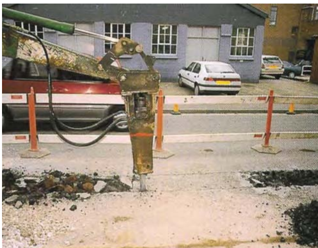
Figure 13.4 Mounted breaker to reduce vibrations.
