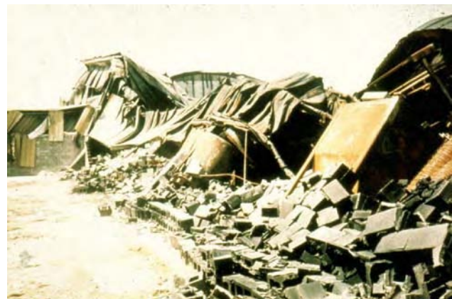
Figure 11.10 Steel structures will collapse in the heat of a fire.
