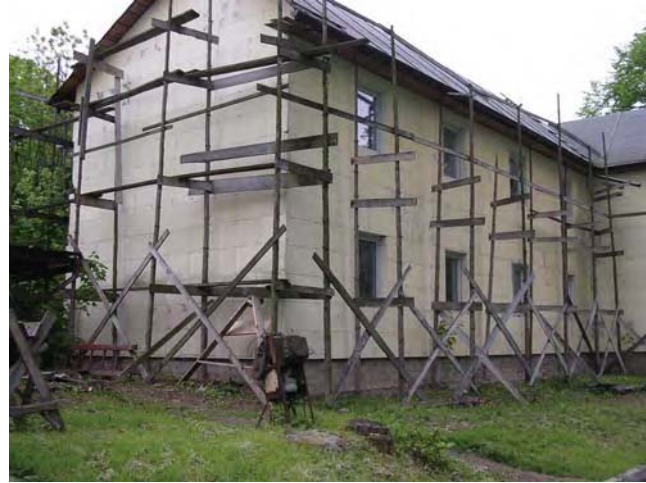
Figure 18.3 Poor standard of scaffold not to EU standards in Poland.
