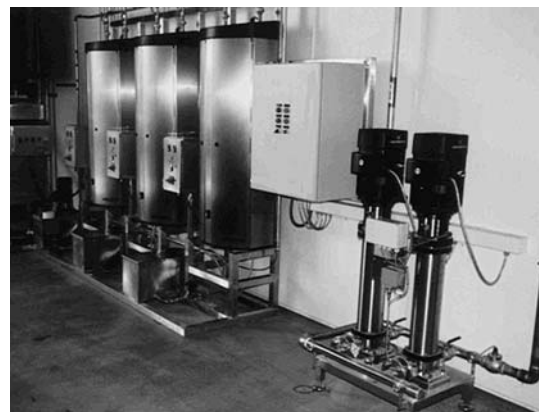
Figure 11–2 A centralized medium pressure, (boosted pressure) system for a large cleaning operation. Courtesy of JohnsonDiversey, Inc., Detroit, Michigan.
