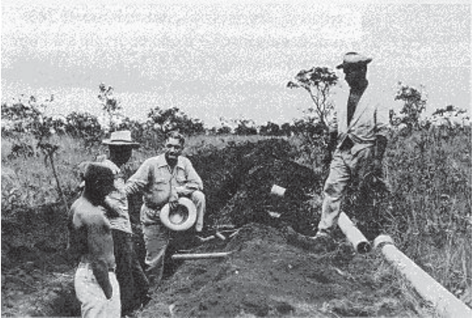
Figure 28.2 Installation of the very first water mains in Brasilia, the new Brazilian capital, in the decade of 1950. (Source: http://www.caesb.df.gov.br/historia.asp , accessed 23/12/2005)
