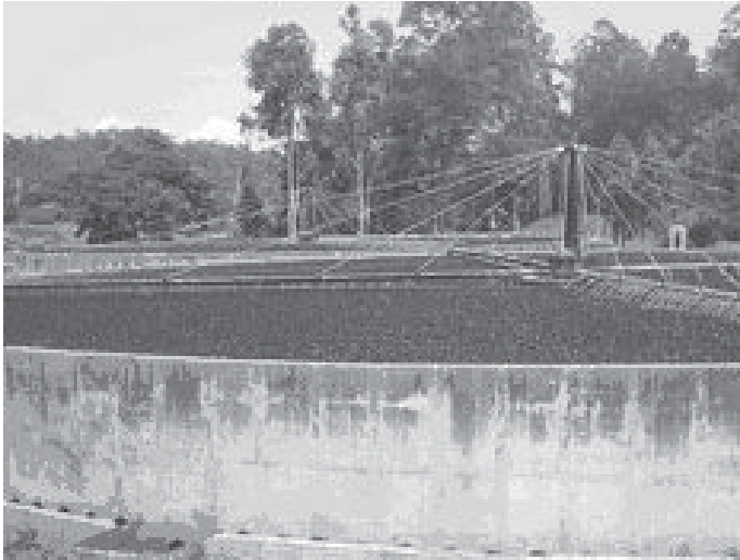
Figure 21.7 Kangemi sewerage works in Nyeri (High rate-percolating trickling filter-commissioned in 1988) (Photo: Ezekiel Nyangeri Nyanchaga)
