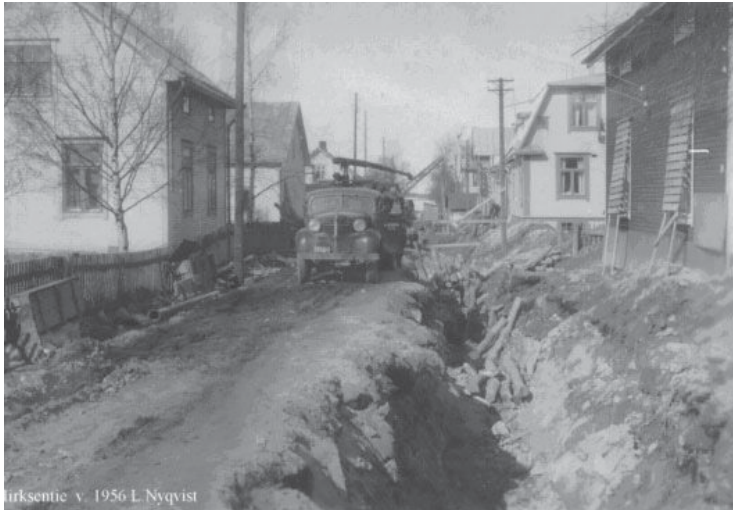
a) Drawing water from a traditional unprotected and open pit in Tanzania in the late 1970s. b) Sewerline construction in the mid-1950s in Vaasa, Finland. (Photo: Vaasa Water)
