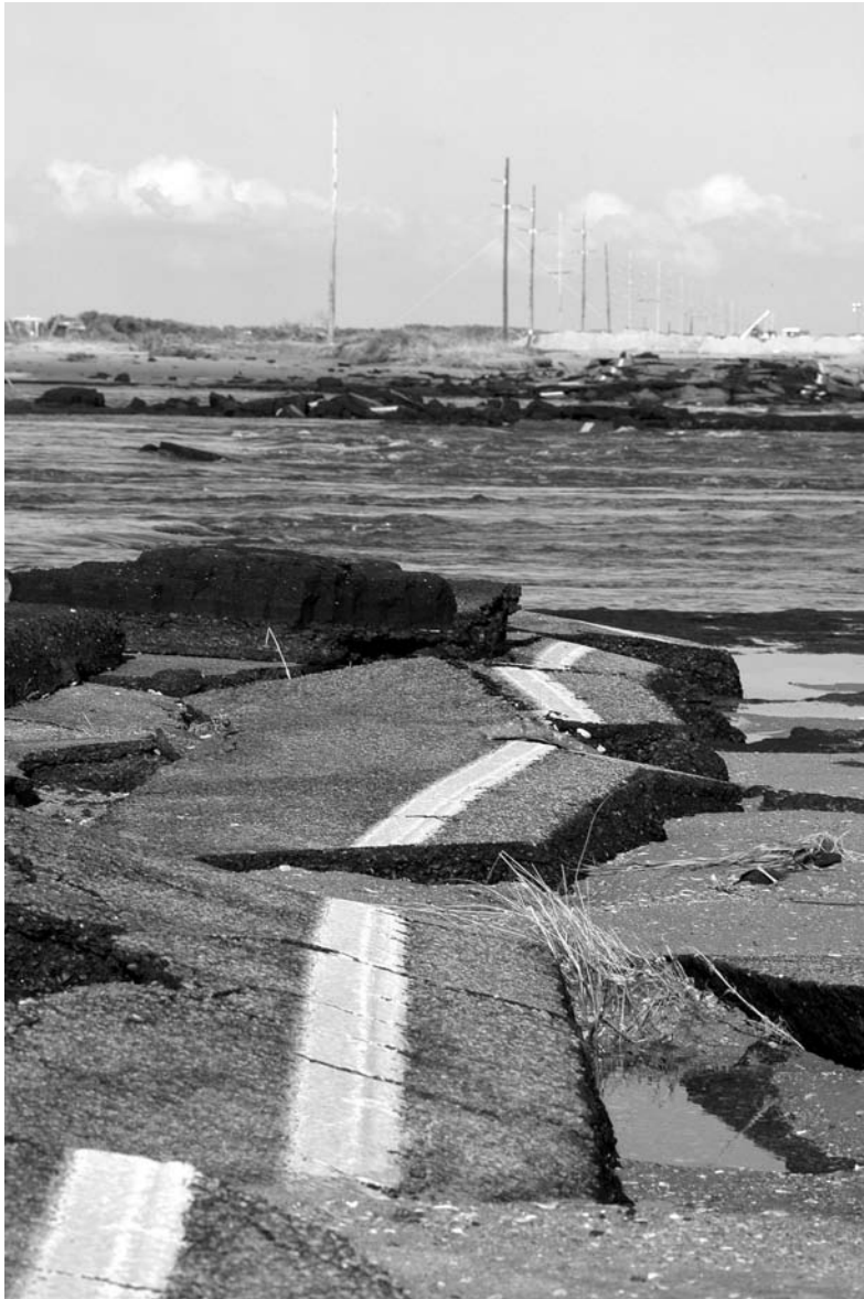
FIGURE 26.3. DESTRUCTION OF NORTH CAROLINA HWY 12 ALONG HATTERAS ISLAND, RESULTING FROM HURRICANE ISABEL, SEPTEMBER 2003.
